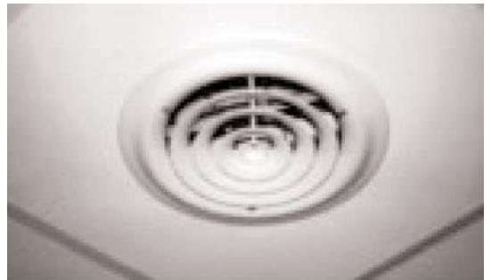
▲ Typical outlet grill
